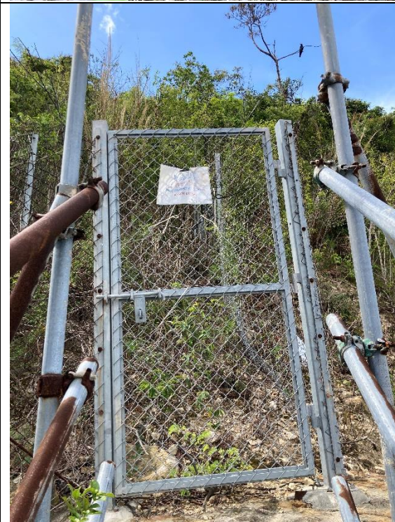
Photo 2 – Current situation of fencing and warning sign
